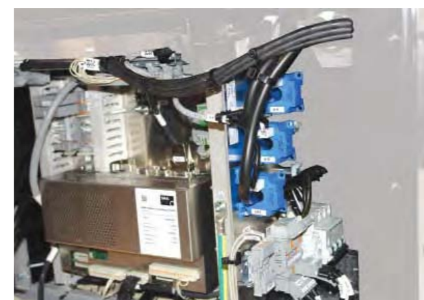
LF 205 models in auxiliary inverter. Picture provided by courtesy of SMA.
